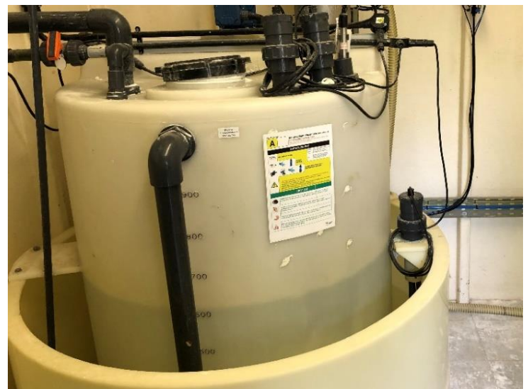
Image 4 Phosphate dosing at a WTW for Plumbosolvency (Lead) Control
