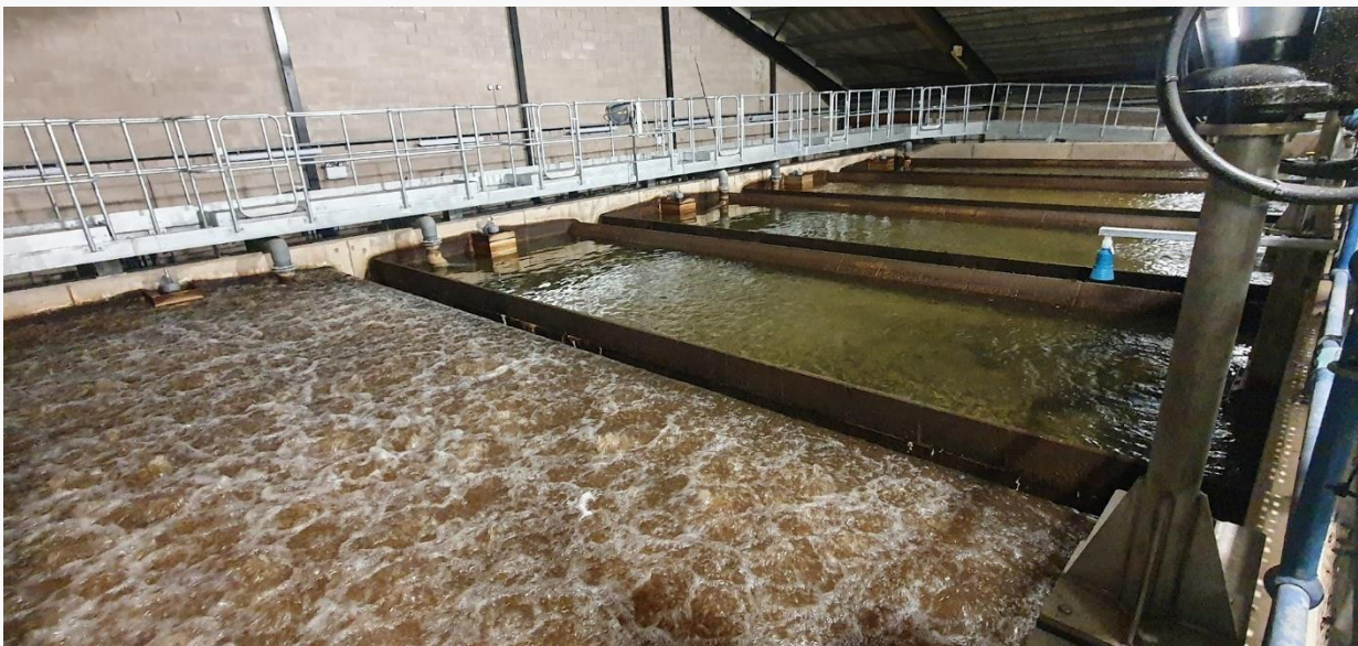
Figure 20 A filter back wash at a WTW
