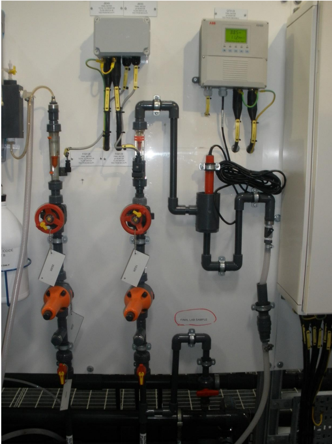
Figure 18 Final water pH monitors at a WTW in the Highland.
