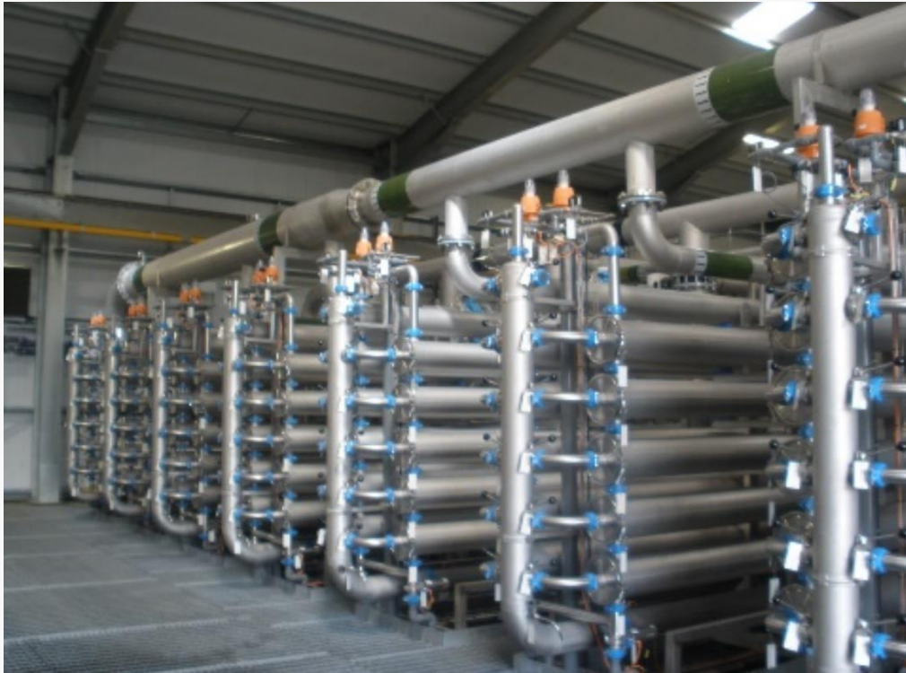
Figure 21 Membrane filters at a WTW
