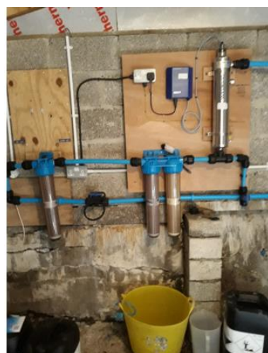
Figure 3 is a smaller private water supply treatment plant.
