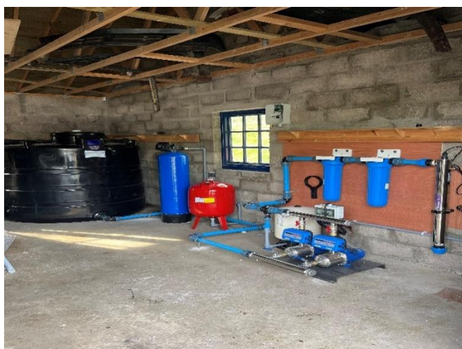
Figure 2 is a larger private water supply treatment plant.
