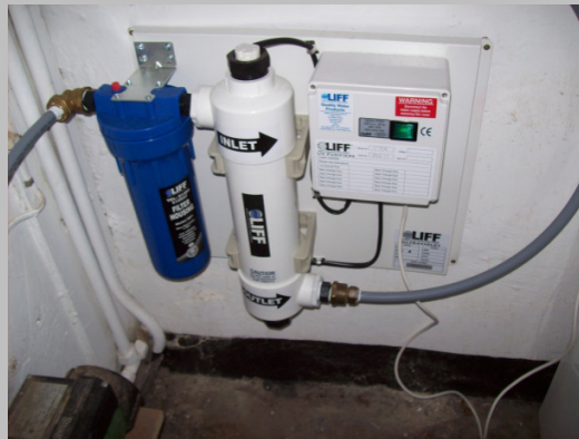
Photo 1: New Point of Entry UV and Sediment Filter
