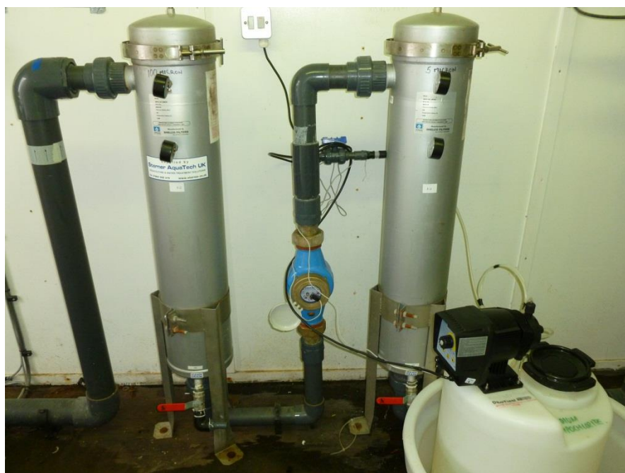
Sequential cartridge filters at 100 micrometre and 5 micrometre, removing particulate matter prior to disinfection with sodium hypochlorite.
