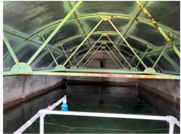
Figure 6 Inside a clarifier in the North of Scotland
