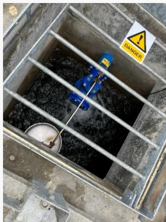
Figure 15 Inspection hatch with secondary chlorine dosing at an SR
