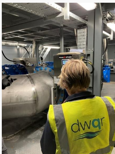
Figure 3 A member of DWQR inspecting a UV unit at a WTW in the North East of Scotland
