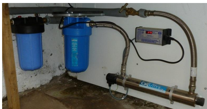
PWS Filtration and UV Disinfection Treatment
