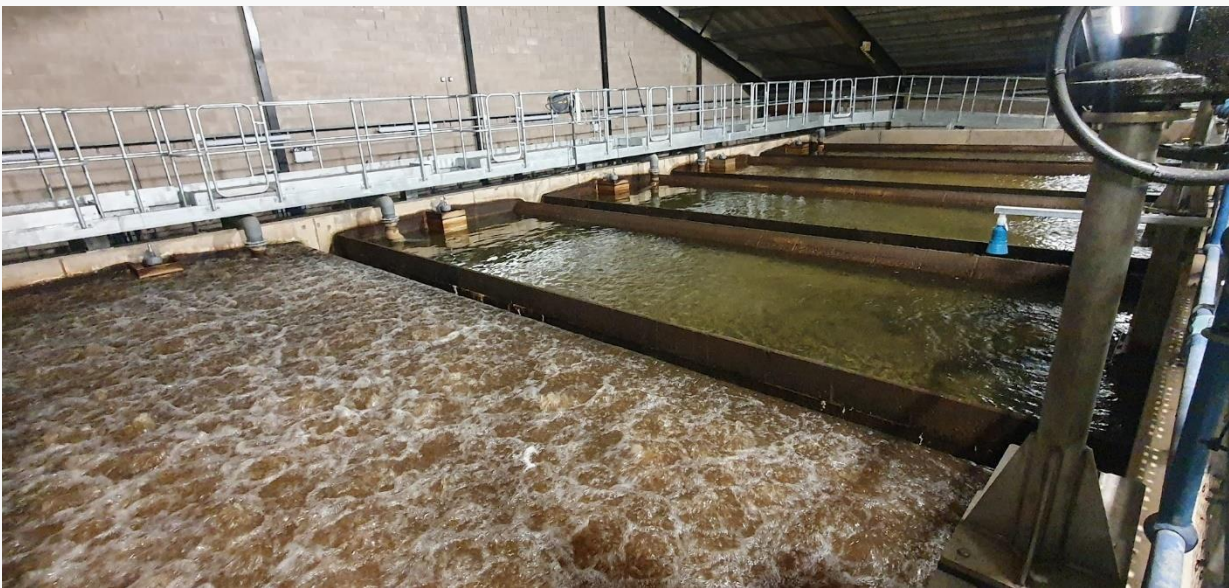
Figure 20 A filter back wash at a WTW
