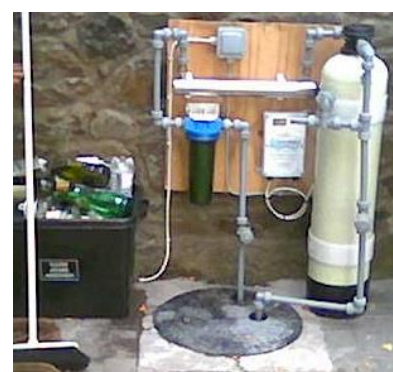
Small Household System with pH Correction - Aberdeenshire Council
