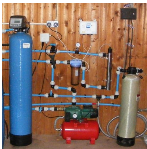
Complex Household System (pH filter is smaller, buff coloured unit) – Aberdeenshire Council
